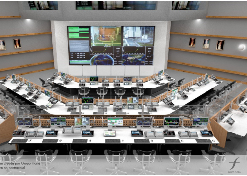
Jupiter Control Centre Realisation
